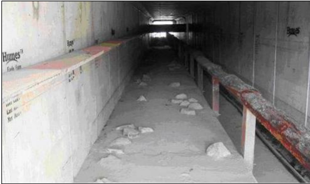
Figure 7: Example underpass design with raised dry access ledge, wooden shelf and log railing (from TMR's Fauna Sensitive Road Design Manual, Vol 2).
